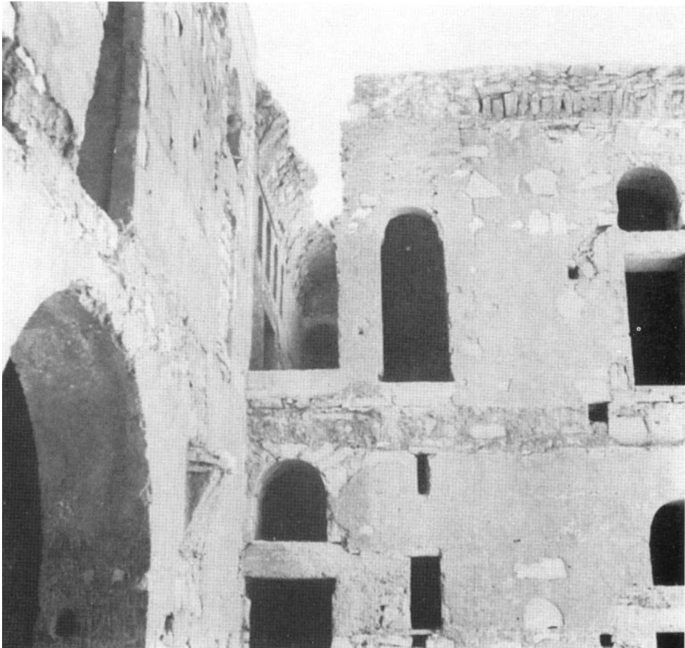
b. The internal courtyard. Note the springing of arches and the traces of a gallery, now disappeared, on the first floor.
